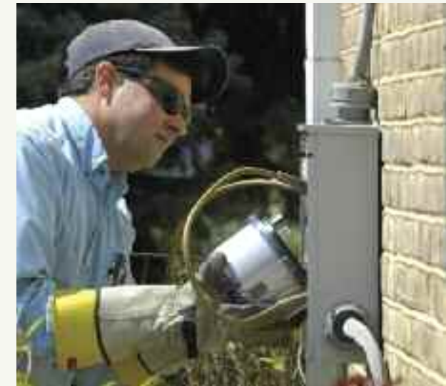
Installing smart meters is one of the first steps toward helping customers better manage their energy use and reduce carbon emissions.
