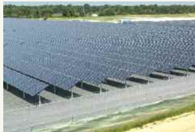
The four MW Vineland Solar One , a key supplier of renewable energy in southern New Jersey, was built and developed by Conectiv Energy.
