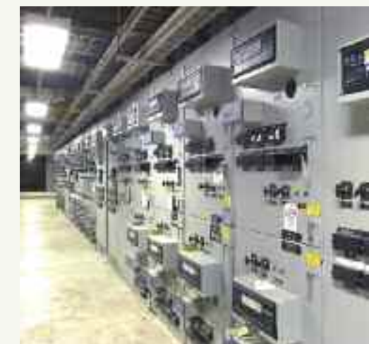
Data is transmitted through fiber optic cable from smart substations like this one to a secure central data point to help customers better manage their energy usage.
