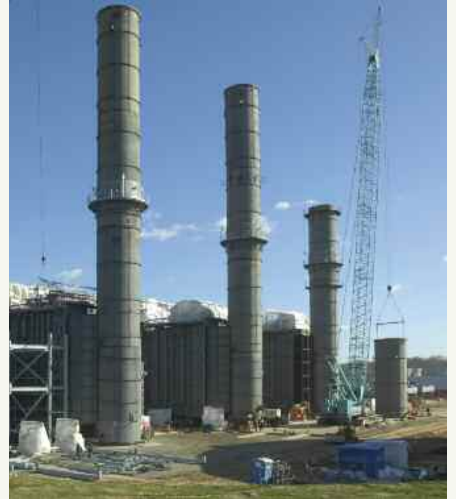
Conectiv Energy's Delta combined cycle power plant will be able to use either natural gas or ultra-low sulfur distillate oil.
